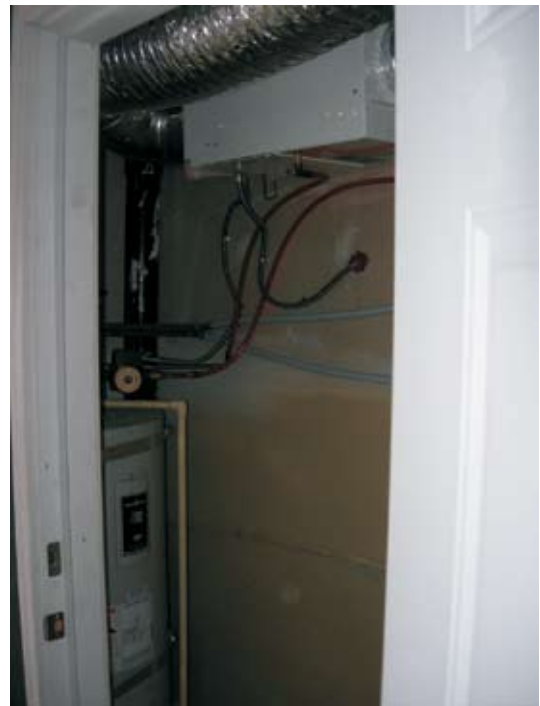
JH unit placed in the closet so very little space was used to provide heating for the suites of this Townhouse
